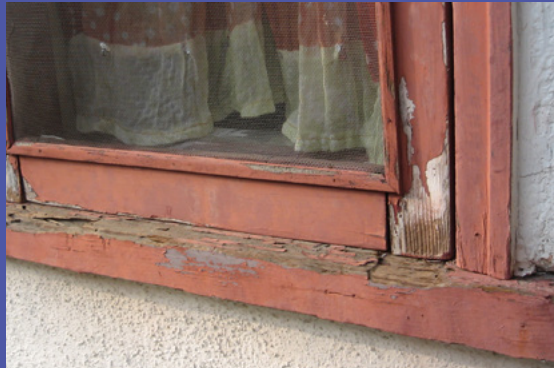
in chipping paint
